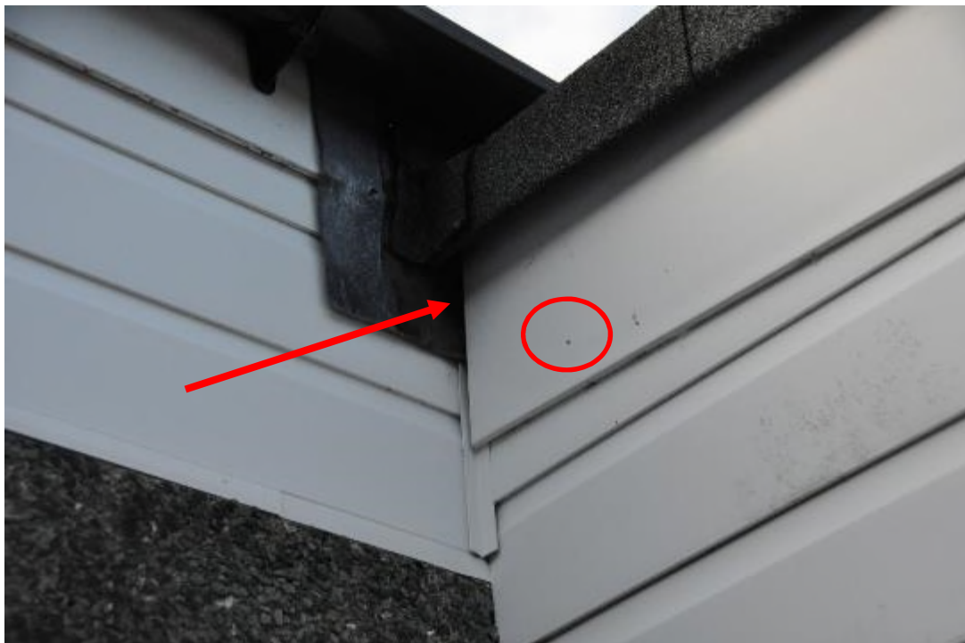
Plate 2 bat dropping recorded on fascia and roost recorded behind lead flashing
