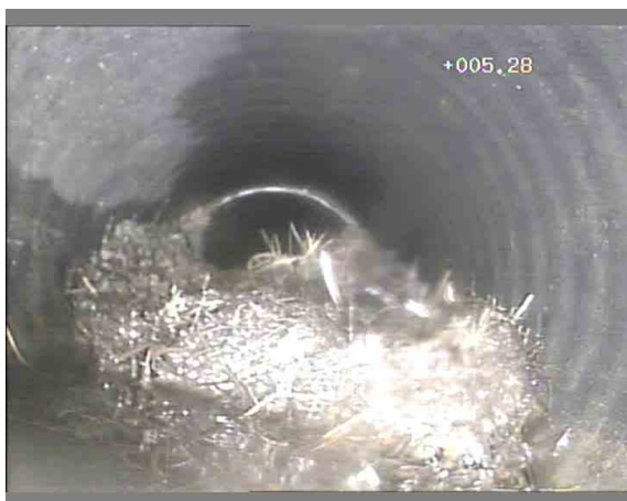
1, 00:00:43, 5.28 m Roots, mass, 35% cross-sectional area loss
