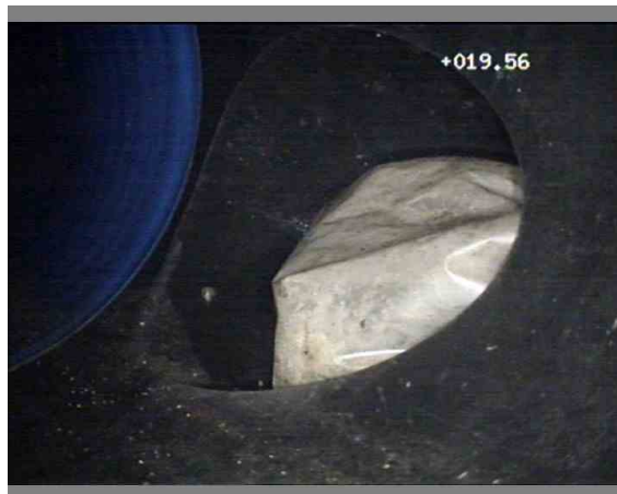
2, 00:04:57, 19.56 m Junction defective, connecting pipe is blocked, at 3 o'clock, diameter 150mm, POLYTHENE WITHIN JUNCTION
