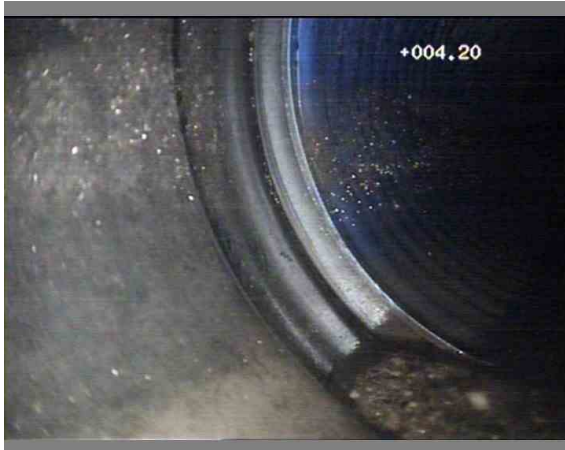
1, 00:01:00, 4.20 m Open joint, large
