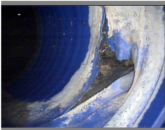
1, 00:03:10, 11.54 m Hole in drain/sewer, from 1 to 3 o'clock
