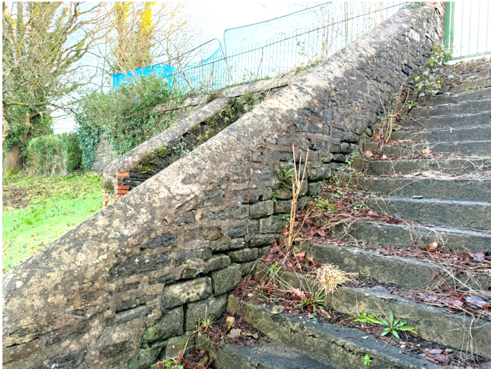
Photograph 14 : Open jointing noted to random stone side walls of access steps.
