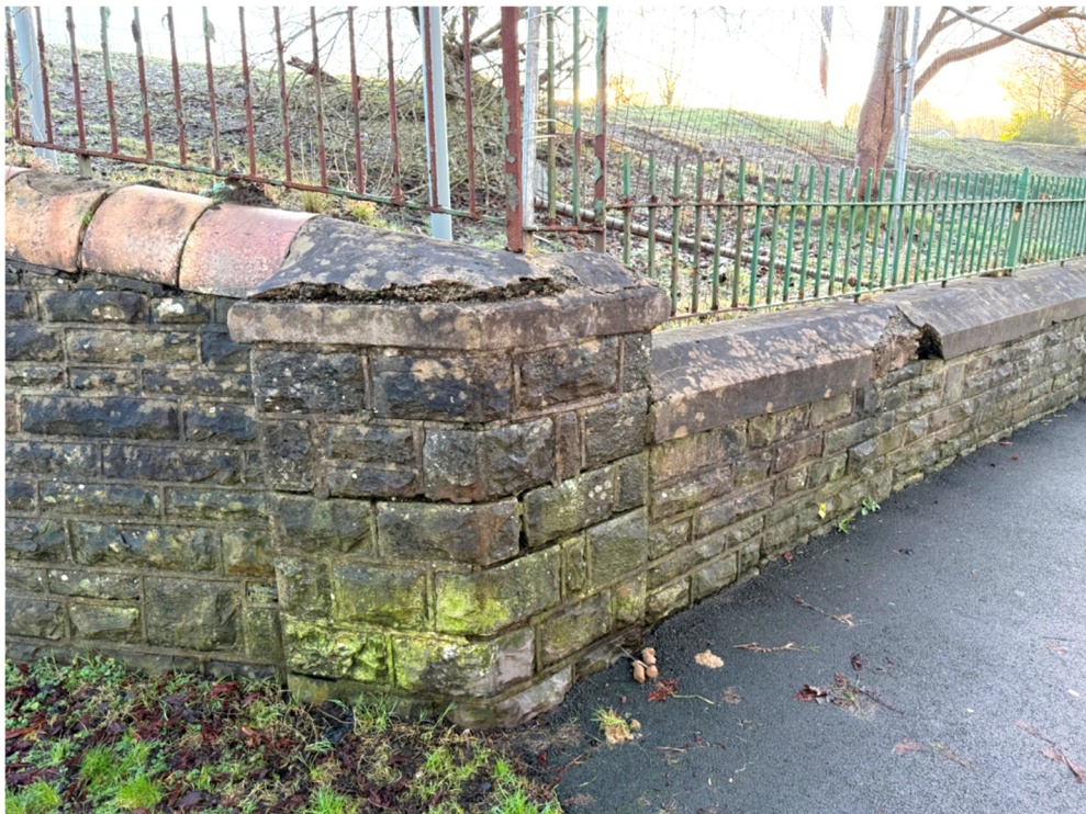
Photograph 22: View at retaining wall corner. Some open jointing but otherwise structurally stable.
