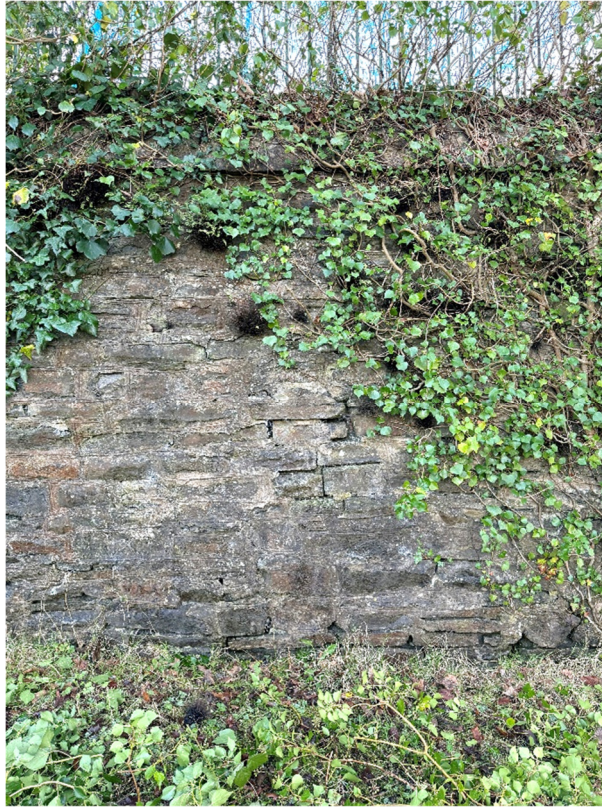
Photograph 7 : Open jointing is noted within the right hand section of retaining wall.
