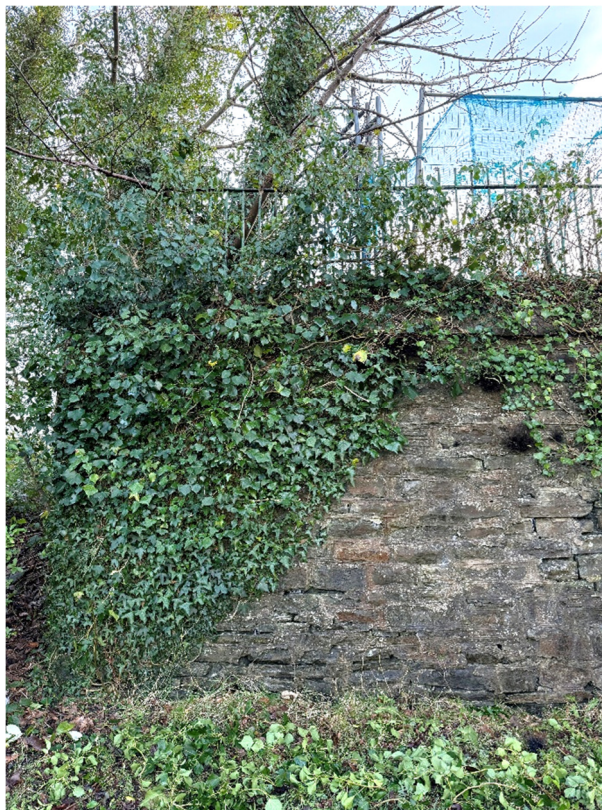
Photograph 6: Ivy has embedded itself into wall joints.
