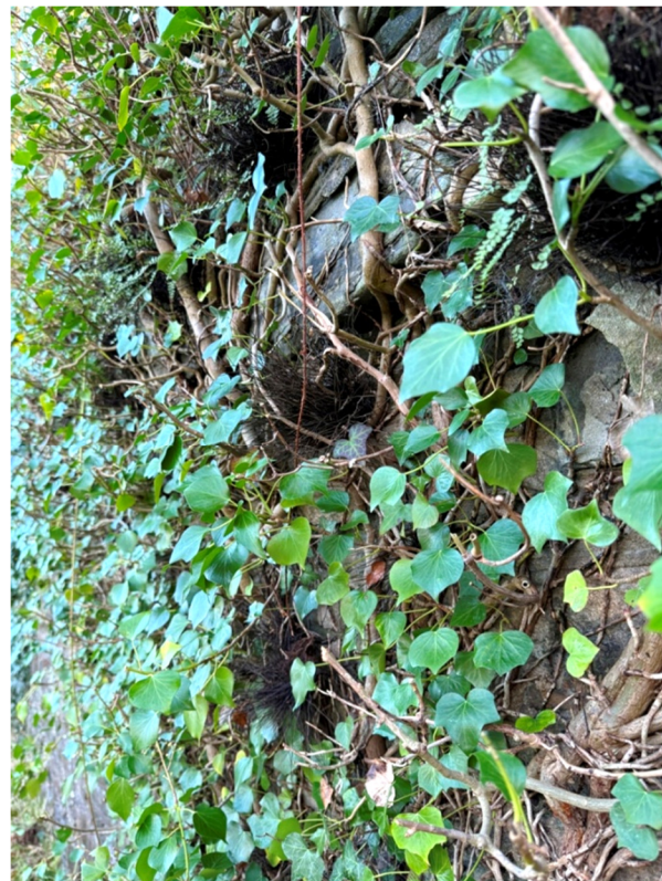
Photograph 8 : Inspection shows displaced stonework approximately 50mm out of line at various locations.
