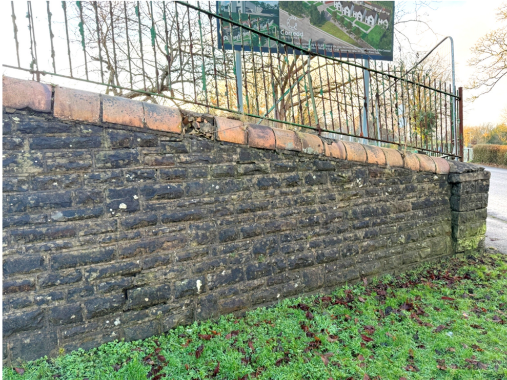
Photograph 21: Minor damage noted to coping stones along the top of the retaining wall.
