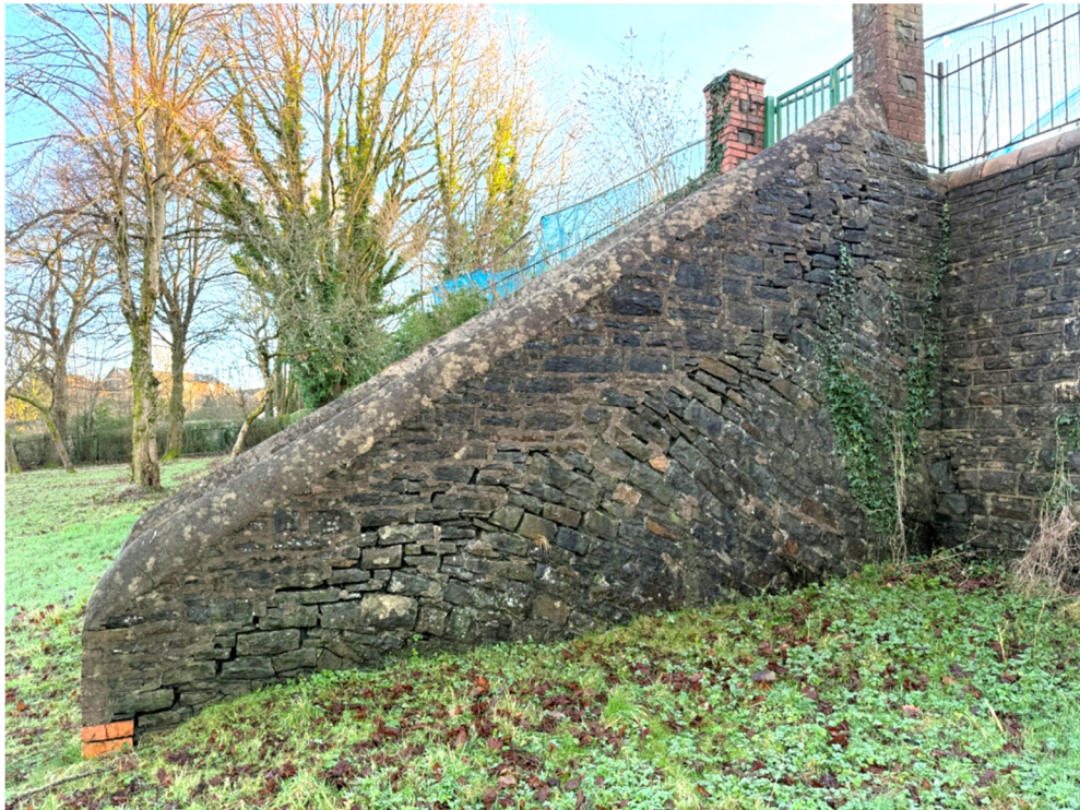
Photograph 16 : Ground levels on the right side of the access steps are lower than the left side.
