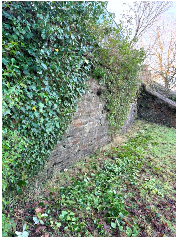
Photograph 5: Retaining wall to right of access steps has a significant forward lean in excess of 150mm.
