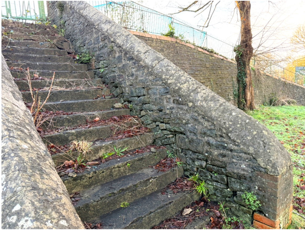
Photograph 15 : View of right hand side wall of access steps. Open jointing noted.
