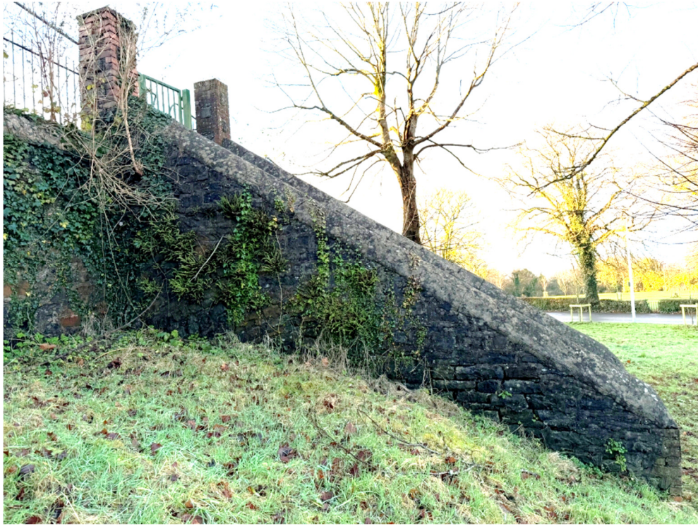
Photograph 13 : View from side of access steps show ground levels raised against the retaining wall.
