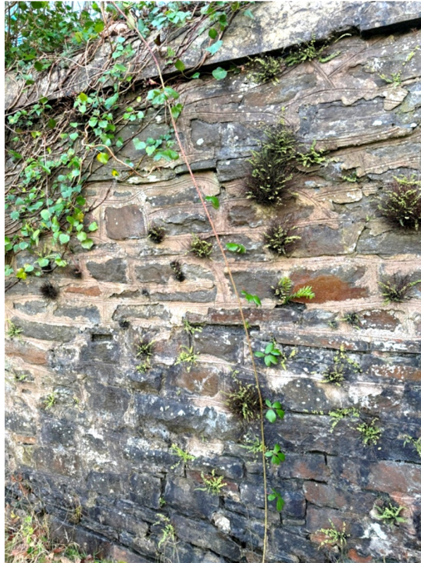
Photograph 9: Another view showing displaced stonework at upper levels of retaining wall.
