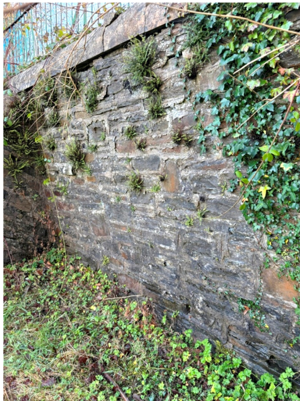
Photograph 12 : View of leaning section of retaining wall in between left buttress and access steps.
