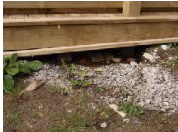
Gap under north west boundary fence
