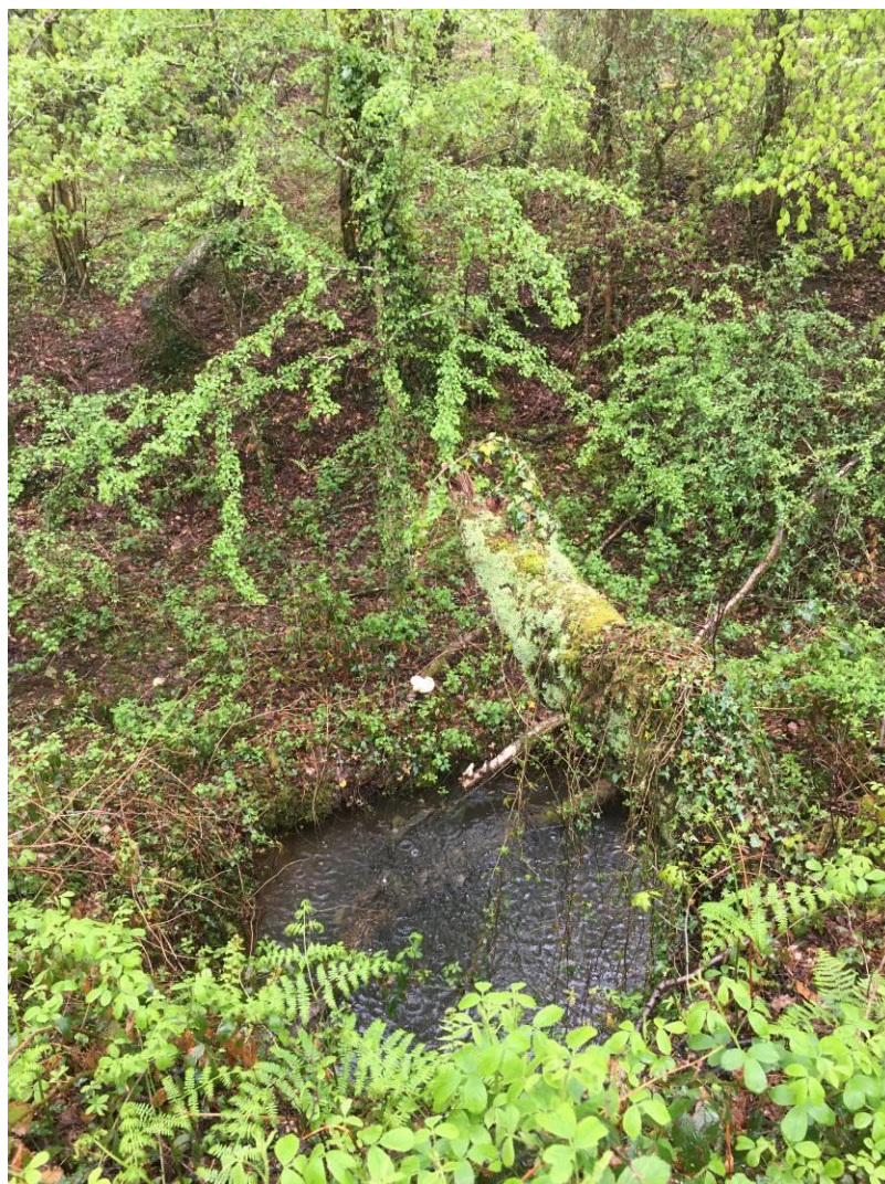
Fig. 4. Area of subsidence within leat & invasive tree/scrub growth (20/05/21)
