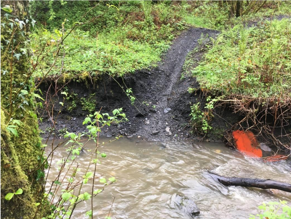
Fig 2. Scour on railway trackbed and erosion from scrambler bikes (20/05/21)
