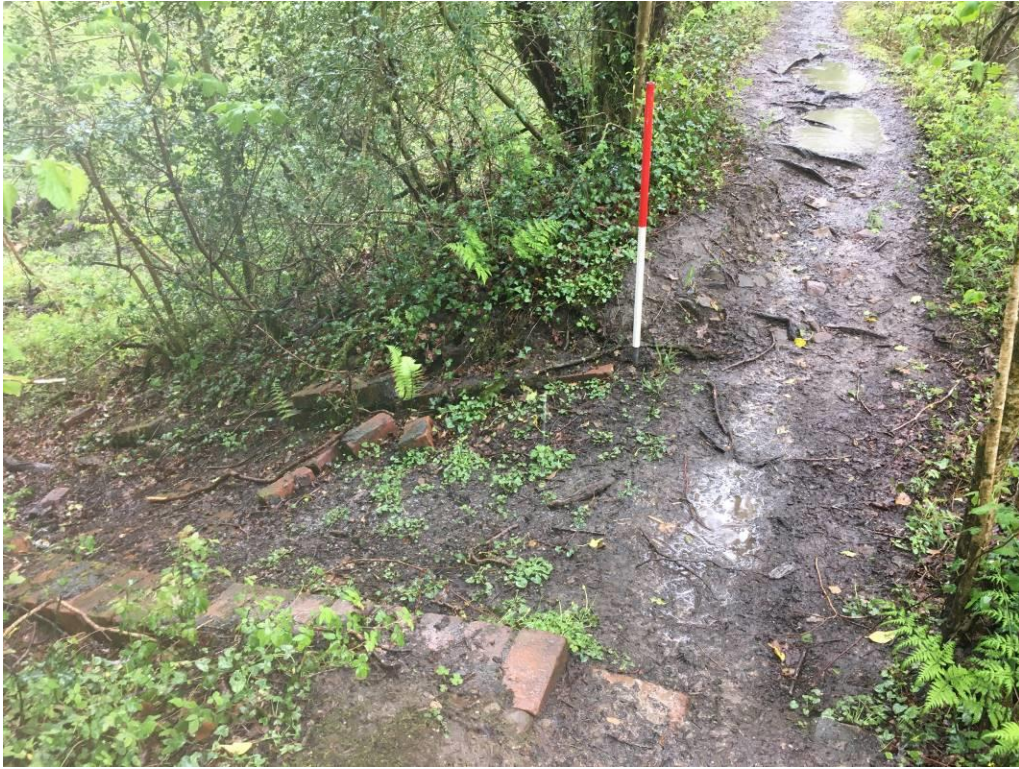
Fig 2. Damage to brick spillway (20/05/21)
