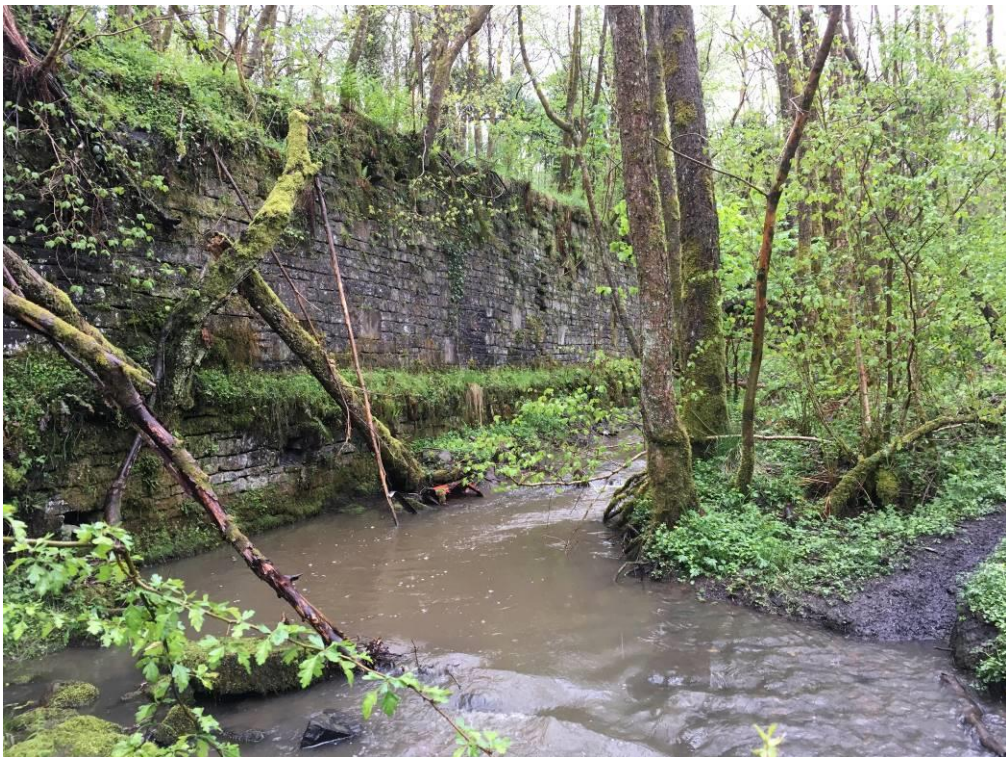
Fig. 3. Vegetation/tree growth on retaining wall and railway trackbed & watercourse (20/05/21)
