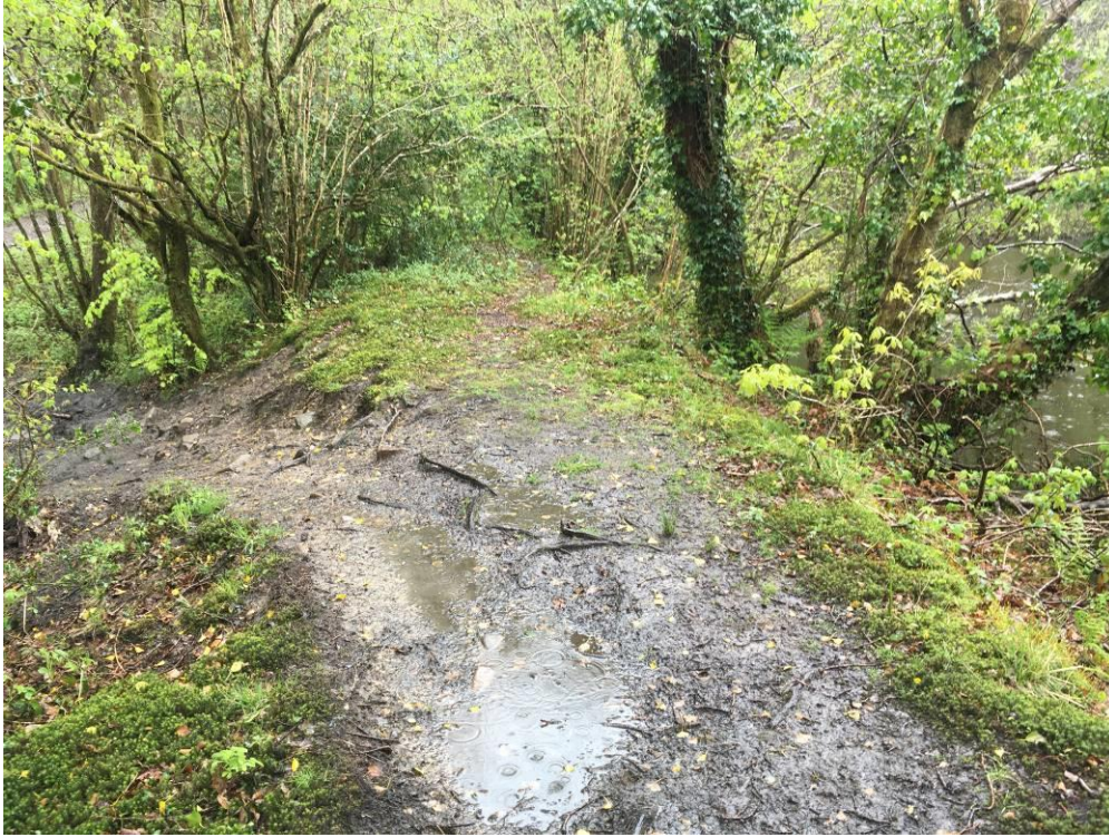
Fig. 5. Path erosion on southern end of pond dam earthwork (20/05/21)
