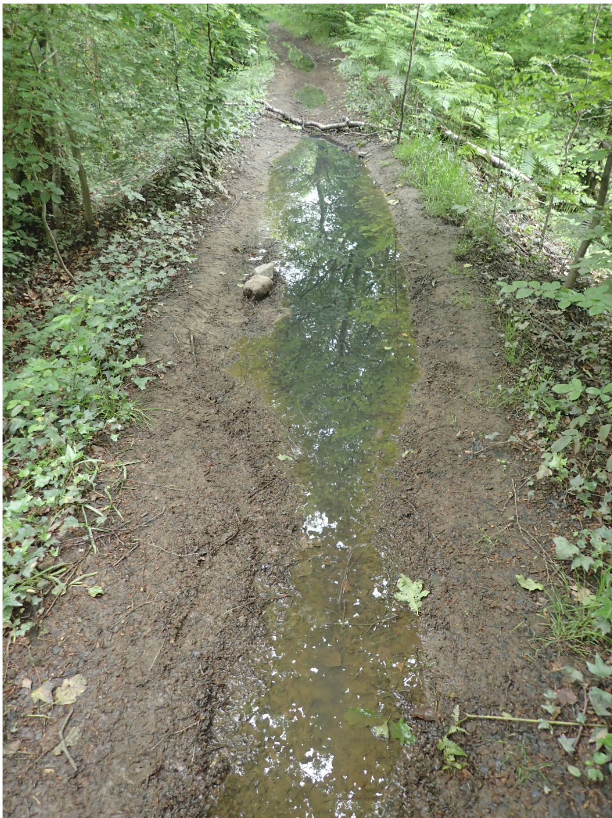
Image EDP 9: Example of one of the many water-filled ruts which line the footpath at the top of the bank at the Pond and Leat.
