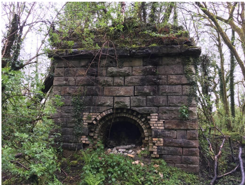
Fig. 4. Chimney stack showing vegetation/tree growth; loose stonework and tree resting on it (20/05/21)
