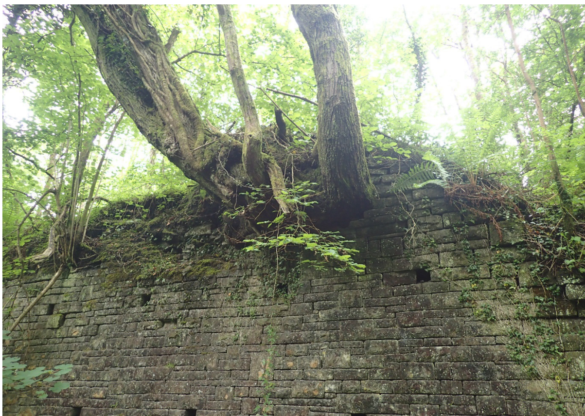
Image EDP 13: Illustration of typical tree damage at the Cwm Pit revetment wall.
