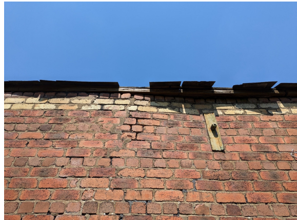
Plate 4: Tiles missing and cracks where mortar missing.
