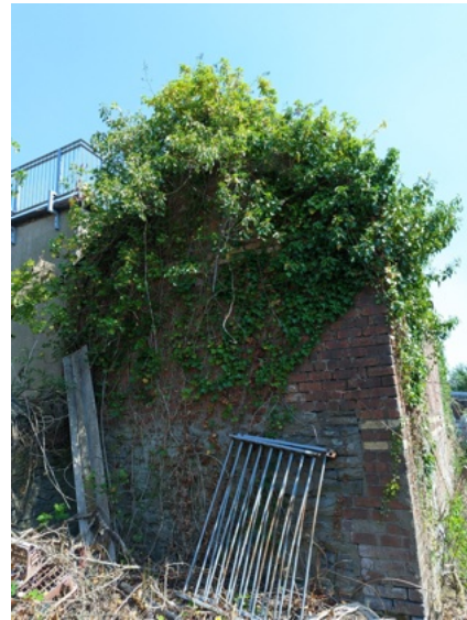
Plate 6: South-west elevation with ivy growing.
