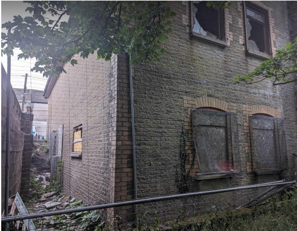
Plate 1- Photograph of rear elevation showing boarded up and smashed windows
