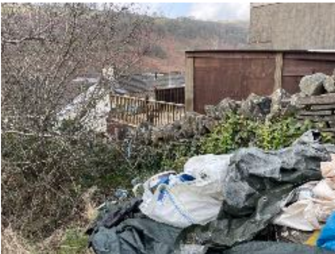
Photograph 3. East boundary wall. With rubbish pile present near top of banking.
