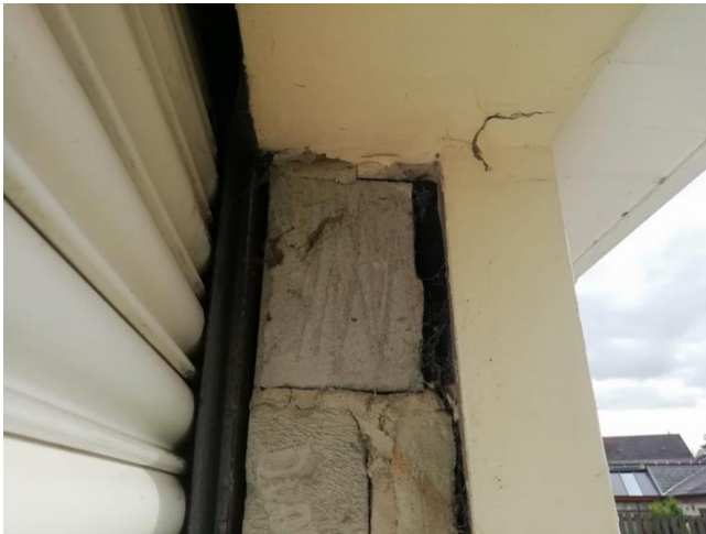
Figure 5 – Roller shutter and gap at block edge on south-western part of garage door
