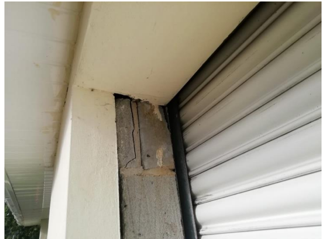
Figure 6 - Roller shutter and gap at block edge on north-western part of garage door
