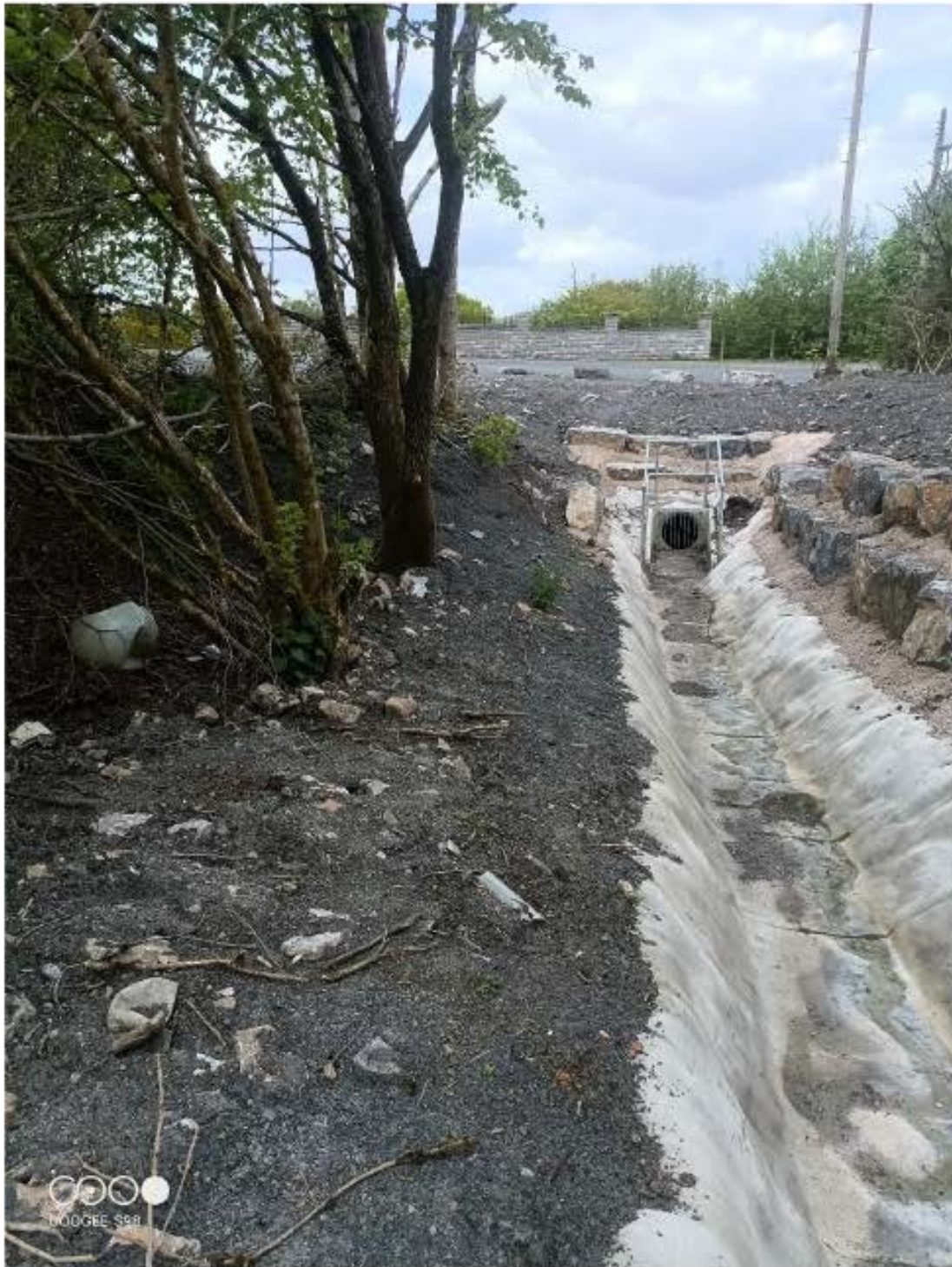
G2 on the left with the new water culvert 1-metre away. All tree roots on this side are now severed. Wind-throw likely
