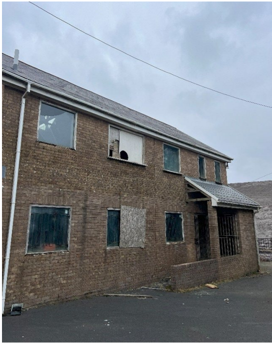
Image EDP A3.7: Derelict Built Structure B4.
