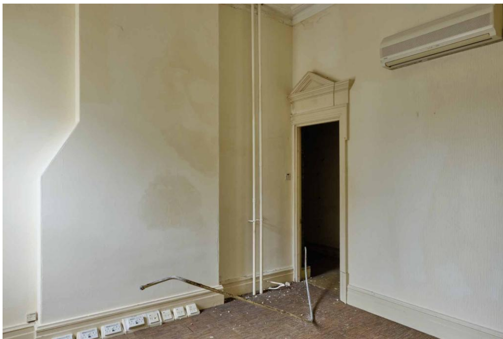
Figure 21. Blocked fireplace in Room 4.
