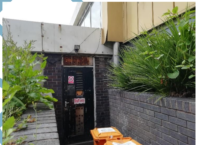
Figure 5 – Joining of the two sections with door with potential holes in (vents)
