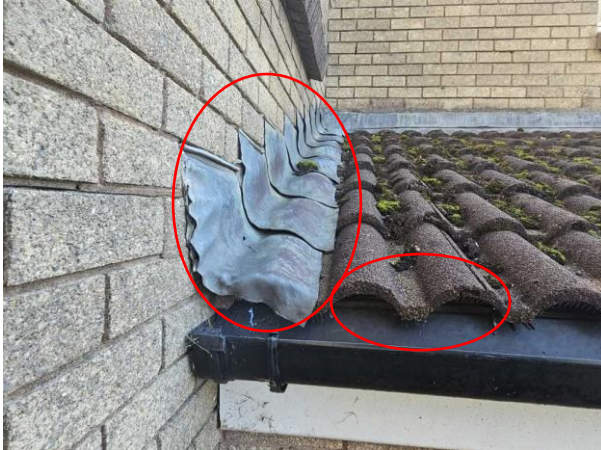
Photo 9: Lifted led flashing and missing wildlife spikes
