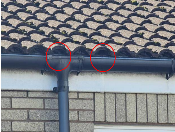
Photo 7: Interlocking tiles with missing wildlife spikes
