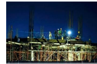
Fig.3.12 – Local task lighting
