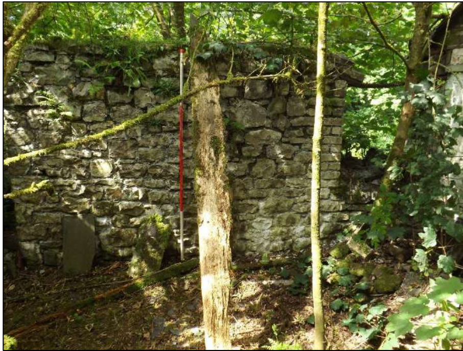
Plate 19. Interior view of annexe 2 showing the west wall and damaged window on the right as well as trees growing in the interior space. Scale 2m.
