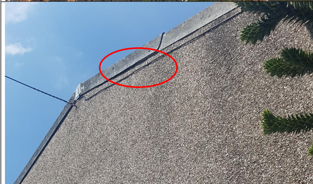
Photo 4. Side gable end (east) with small gaps at the barge board. Possible bat emergence point highlighted.
