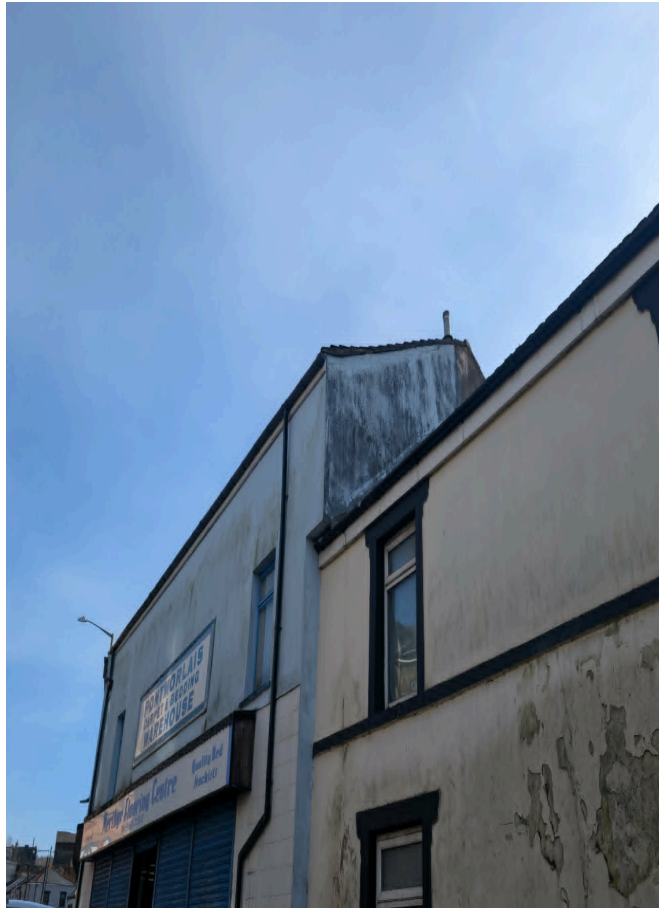
Plate 5 – Photograph of gable end of 13 showing tight fitting cement
