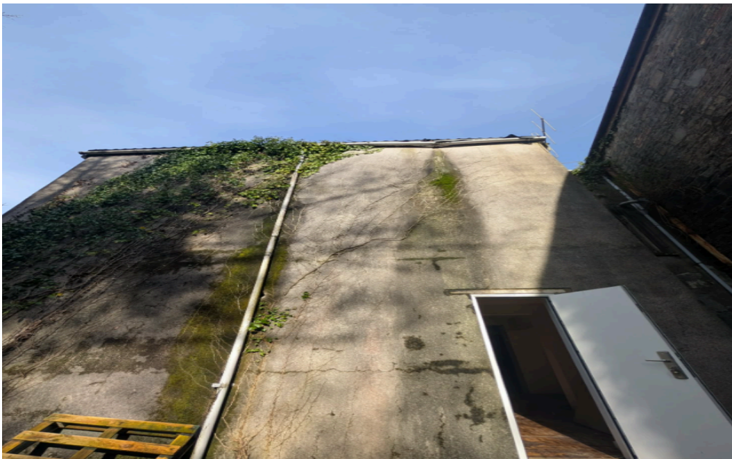
Plate 6 – Photograph of rear two storey extension with snapped guttering
