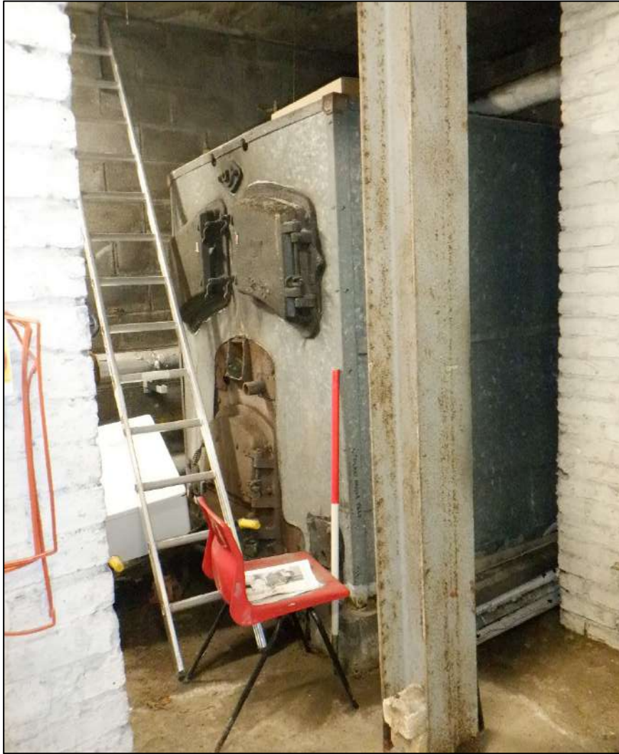
Plate 12: Existing boiler, looking east. 1m scale.
