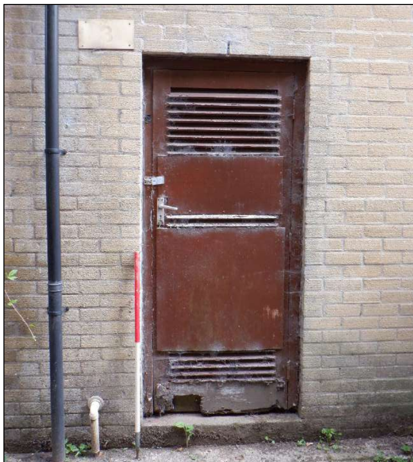
Plate 8. Boiler Room door, in poor condition. Looking north-east, 1m scale.
