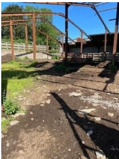
Photo 1 – Shell of fire damaged agricultural shed prior to being re-built
