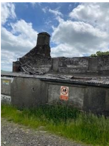
Photo 7 – health and safety signage to prevent entry to burnt out and dangerous old farmhouse.
