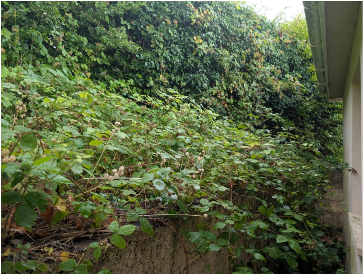
Plate 6- sealed eaves and retaining wall at rear
