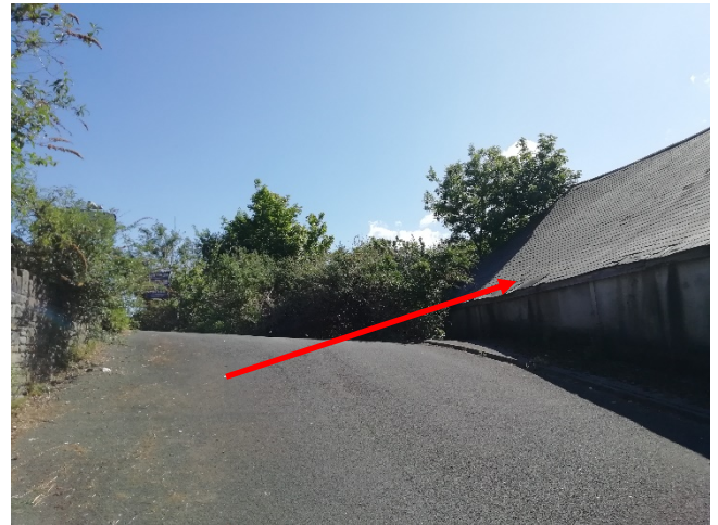
Figure 9 – Northern aspect of the building (arrow showing slipped slates)
