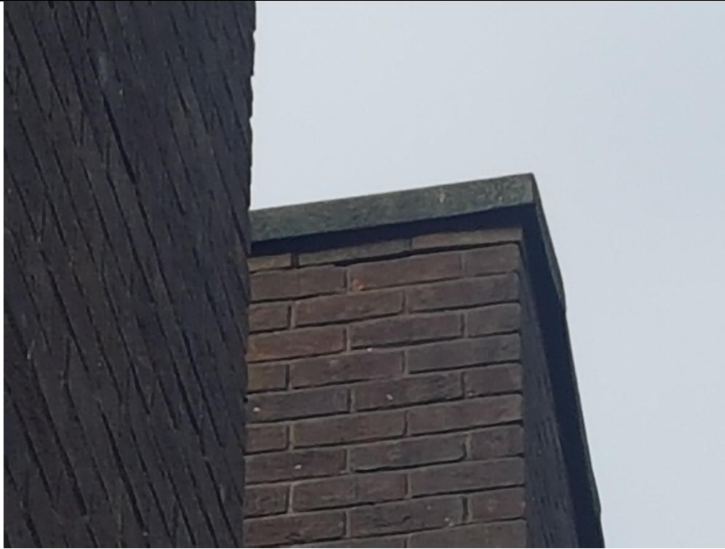
Photo 7. Gaps around roof edge to northeas t corner
