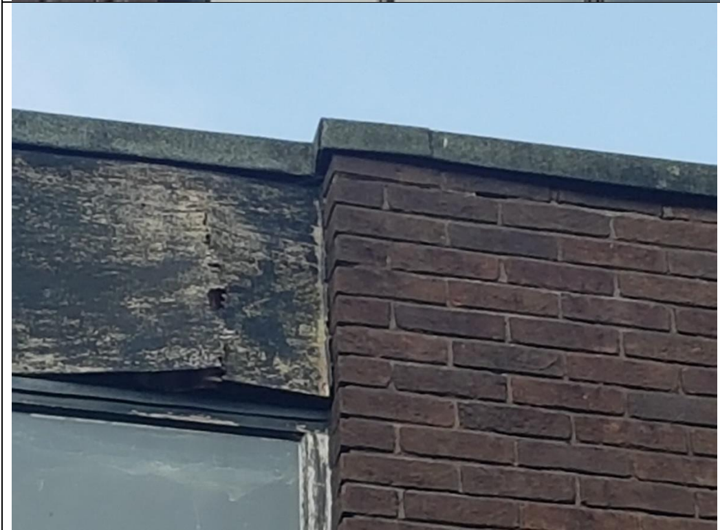
Photo 6. Gaps and roof edge and board to east
