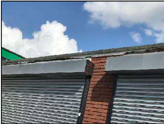
Warped barge boards above the roller doors on the main school building.
