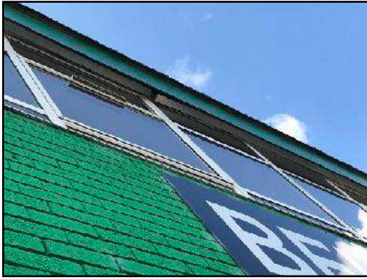
Dislodged fascia board on the west elevation of the main school building.
