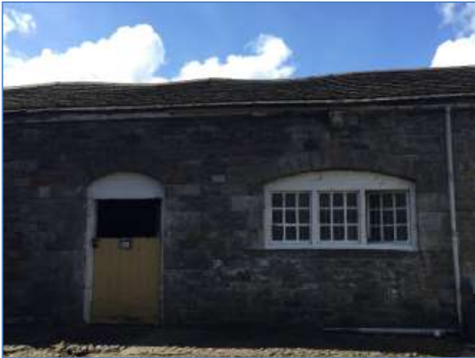
Photograph 37. Building H. The northern elevation showing bowing of the roof and an open stable door.
