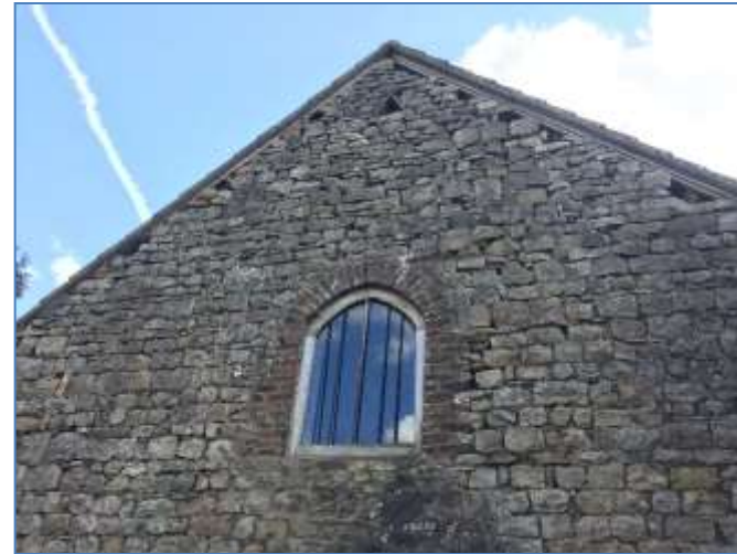
Photograph 10. Building B, western section. Gappy verges on the western elevation.
