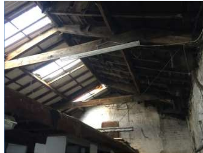
Photograph 38. Building H. The internal space showing northern pitch of roof in very poor condition.
