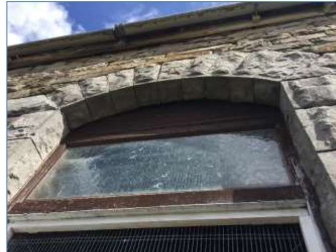
Photograph 28. Building F. Gaps present below window arches.
