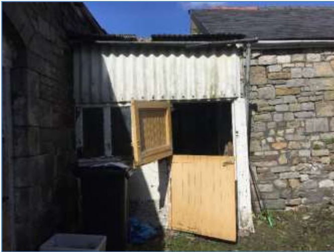
Photograph 17. Building D. The damaged storeroom entrance on the eastern elevation.
