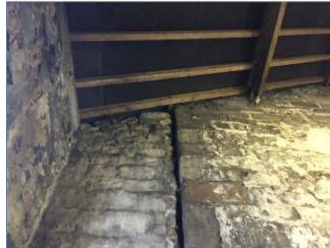
Photograph 36. Building G. A large internal crevice and the bitumen felt in good condition in close proximity to where bat droppings were recorded.
