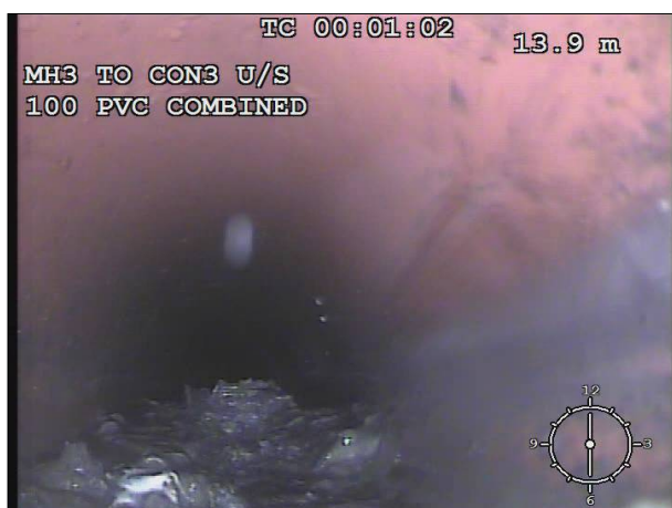
Photo: 49_8a, 00:00:00 13.9m, Debris, 40 % cross-sectional area loss
