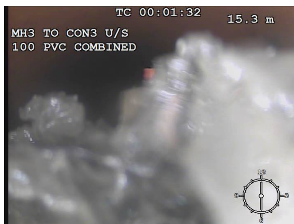
Photo: 50_9a, 00:00:00 15.3m, Survey abandoned, Remark: Unable to CCTV past debris
