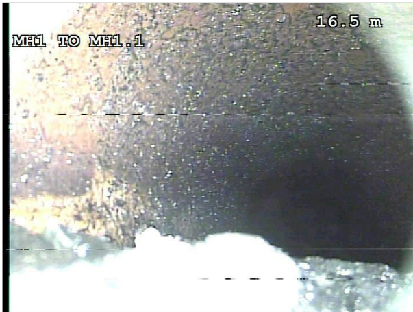
Photo: 59_8a, 00:00:00 16.5m, Debris, 20 % cross-sectional area loss
