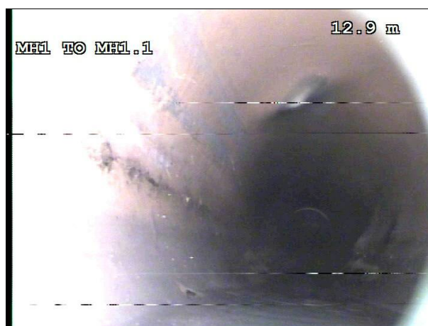
Photo: 58_7a, 00:00:00 13.2m, Sewer Deformed, 10 %, Remark: Stone Impact, from 11 to 01 o'clock
