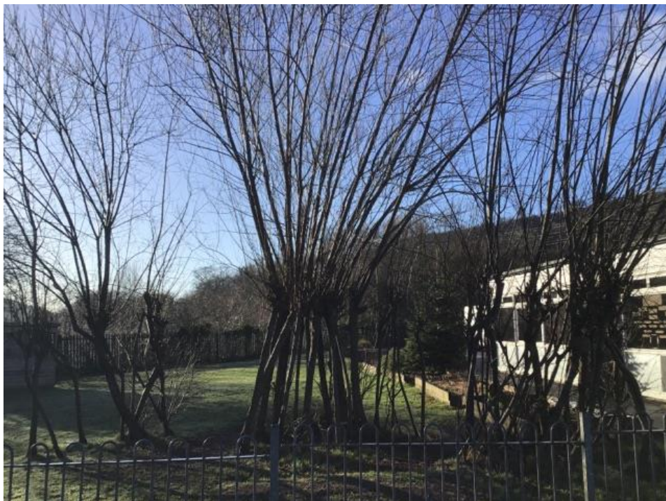
Image 3: Willow structure to the rear of the Building needs reducing and re-weaving to reform structure.
