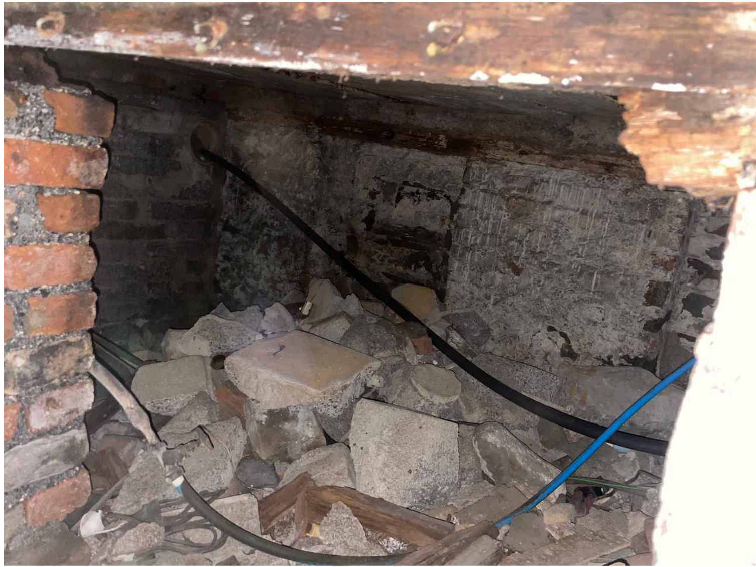
Image Showing Existing Moniques Basement Party Wall NTS
