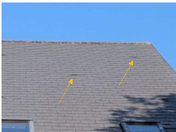
Building A (Former Church): Exterior – South-eastern elevation – minor lifted tiles likely with gaps too small to support occupation but bats.
