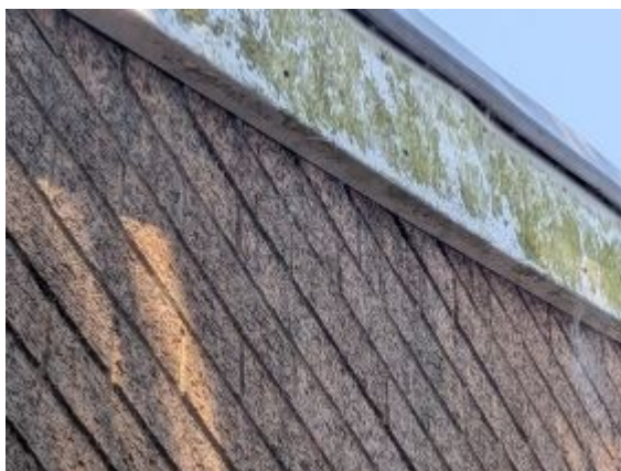
Building A (Former Church): Exterior – North-eastern elevation – Minor gaps between uPVC Bargeboards and brick surface likely too small to support occupation but bats.
