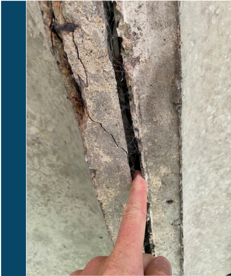
Example crack underneath the bridge - 15mm x 20mm
