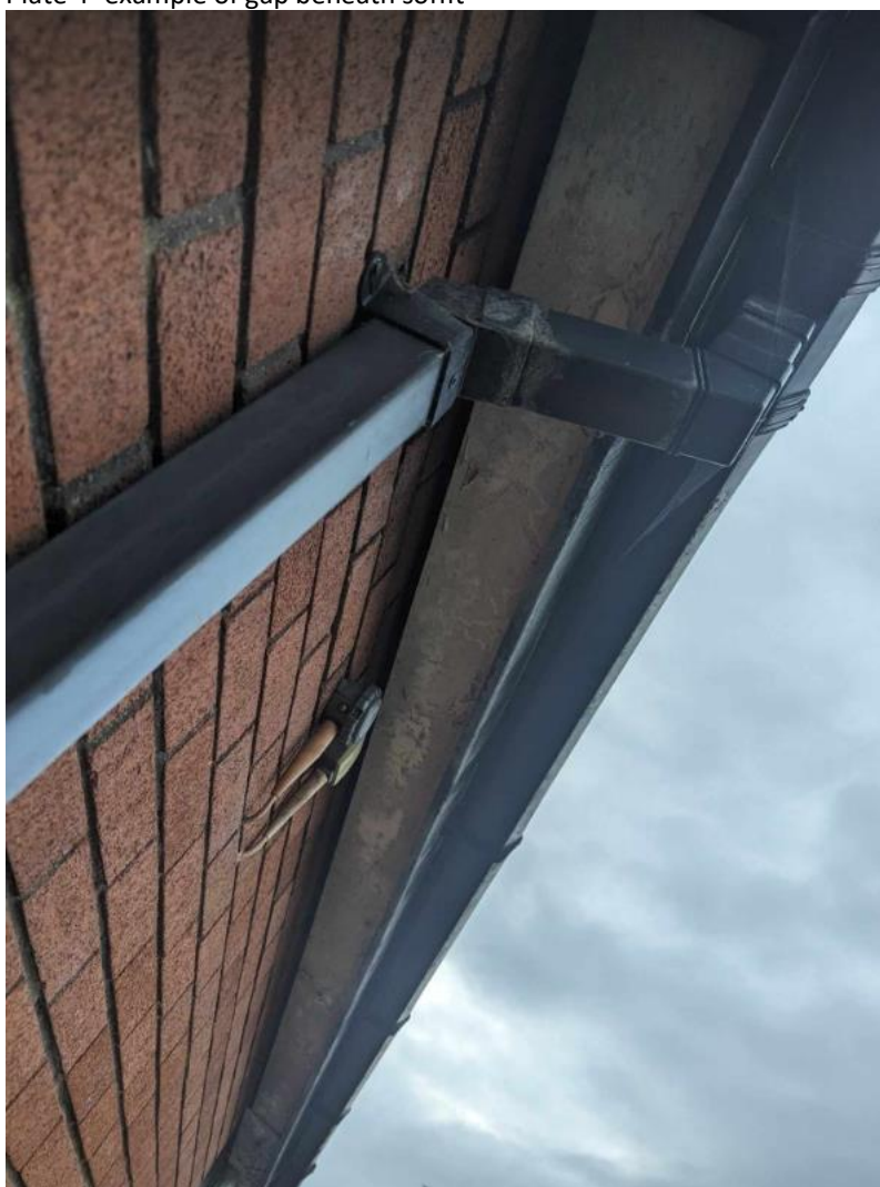
Plate 4- example of gap beneath soffit
