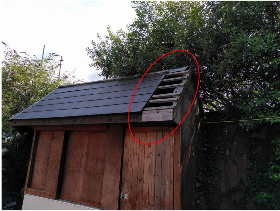
Figure 1 – missing slate on store structure.
