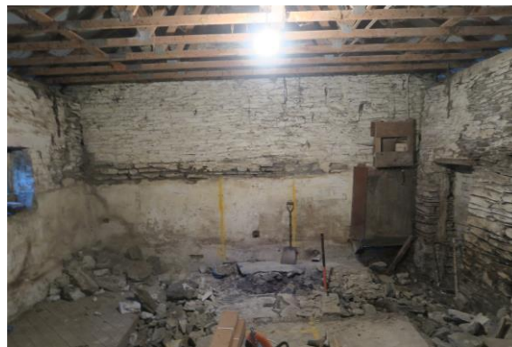
SOUTH ELEVATION INTERNAL: NOTE BOARDED OVER OPENING AND WITH STRAIGHT JOINTS AT CORNERS:
