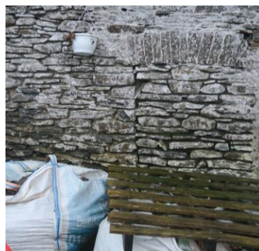
EAST ELEVATION / SOUTH END: NOTE INFILLED OPENINGS WITH STRAIGHT JOINT:
