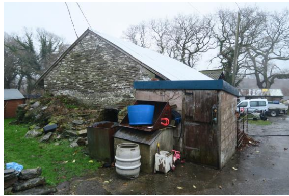
NORTH ELEVATION: NOTE RUBBLE AGAINST WALL AND PALER BAND OF STONE – STRUCTURE AT CORNER TO BE REMOVED:
