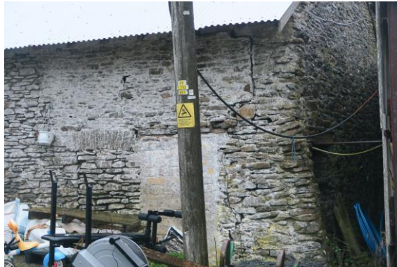
EAST ELEVATION / SOUTH END: NOTE INFILLED OPENINGS AND CRACK IN UPPER SECTION:
