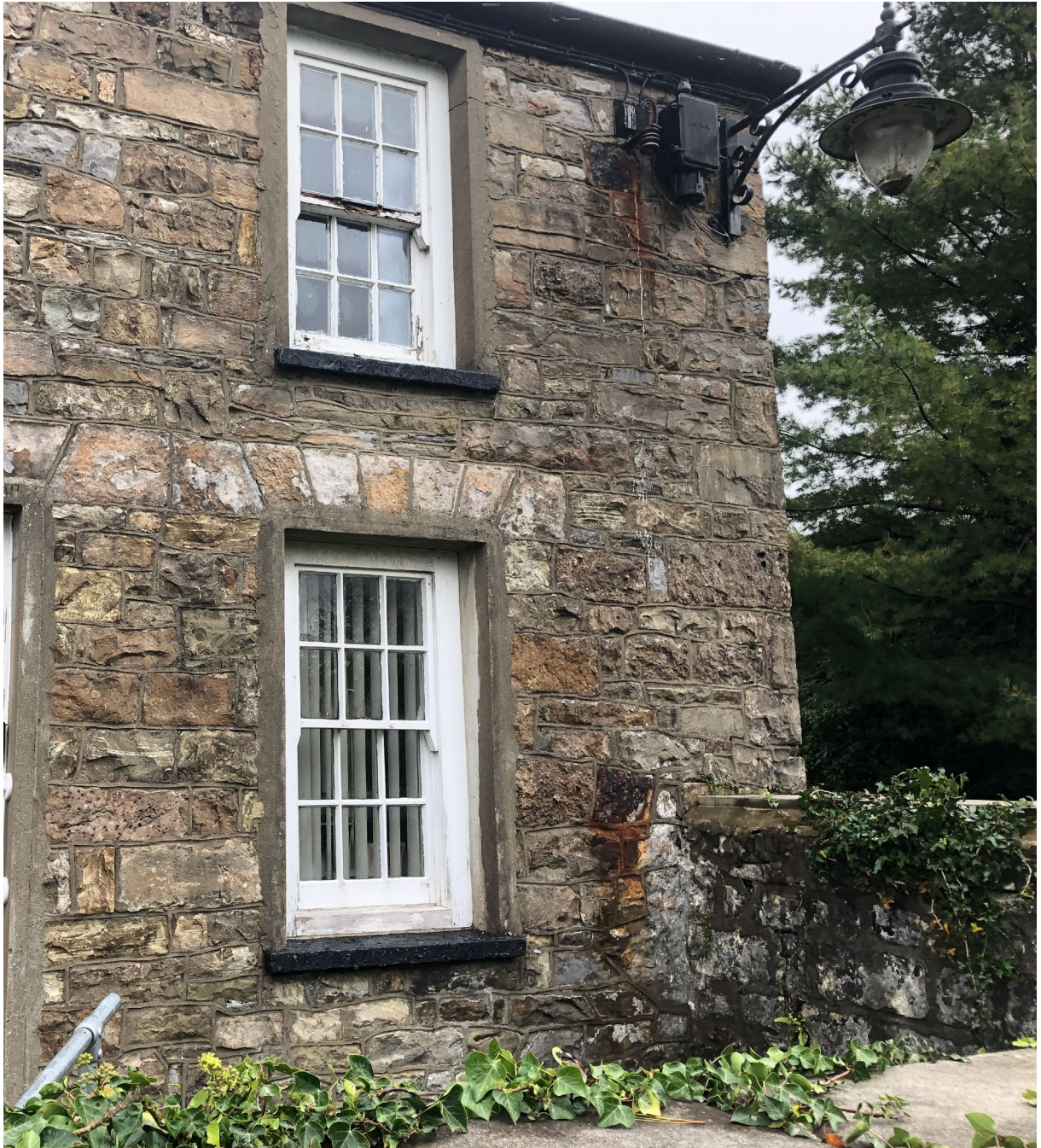
Photo 3 – Windows – First floor window in poor condition
