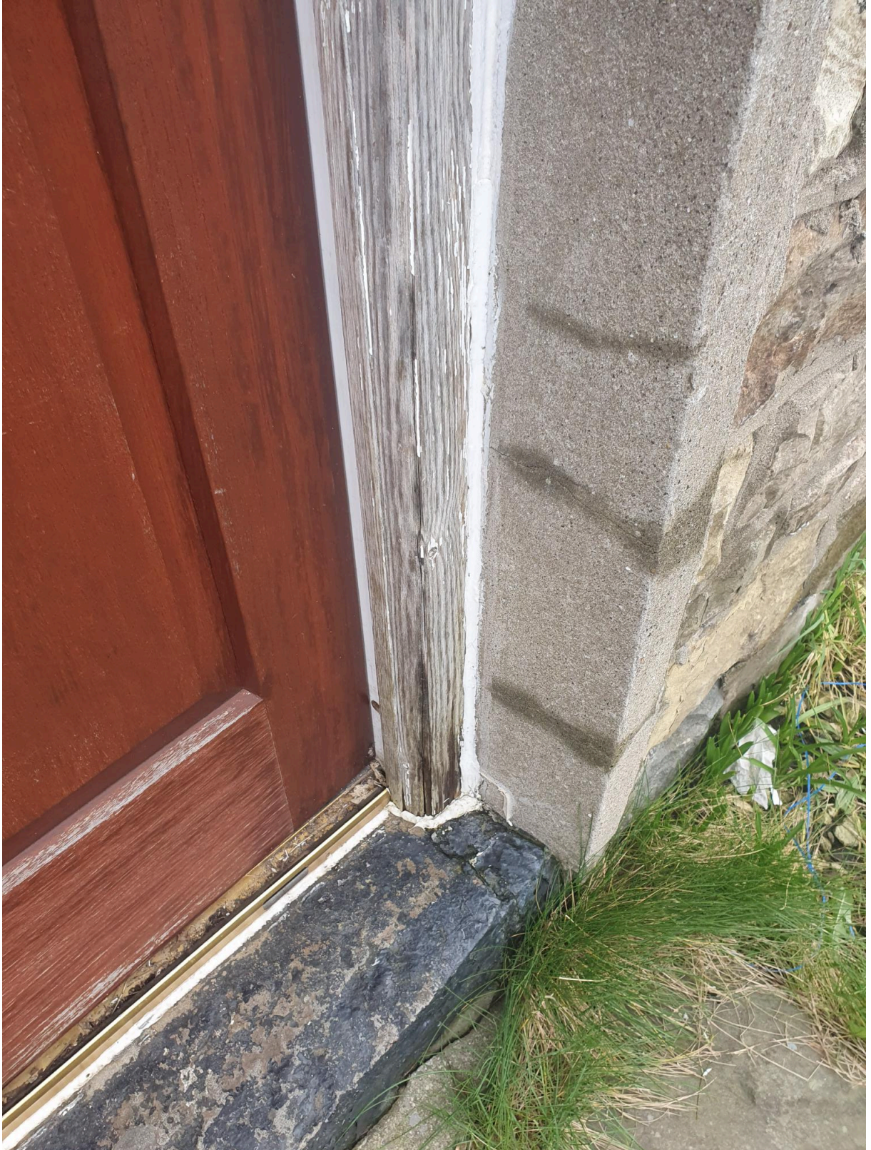
Photo 4 – Front door – rot to the base of the door frame
