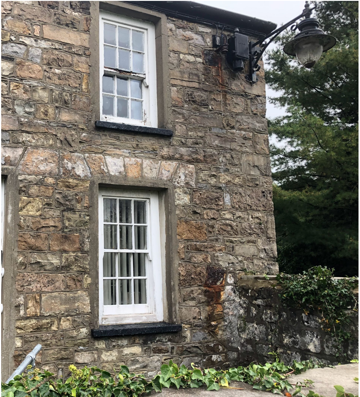
Photo 4 – Windows – First floor window in poor condition
