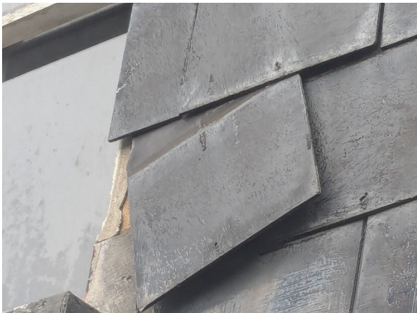
PRFs – Raised/slipped slates.
