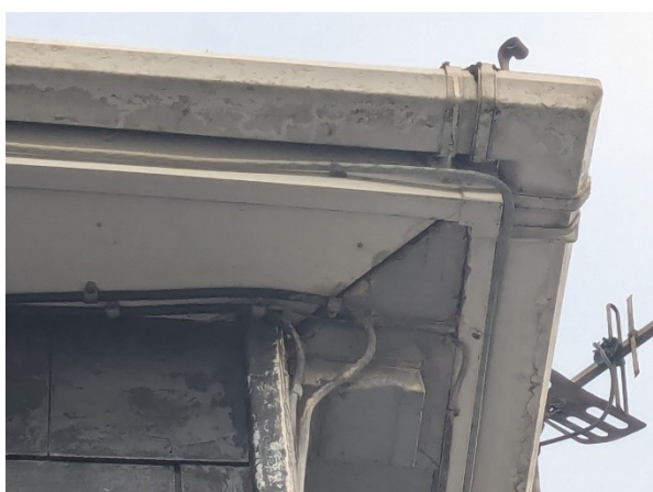
PRFs – Gaps in soffits.
