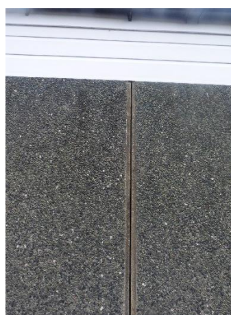
Photo 10: Gap in concrete cladding on eastern aspect
