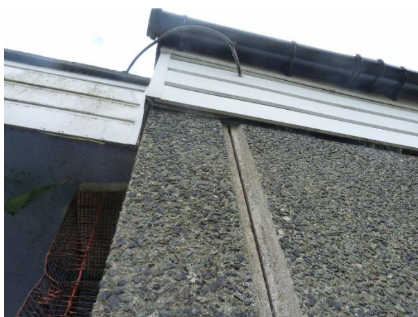
Photo 9: Gaps under uPVC fascias on eastern aspect
