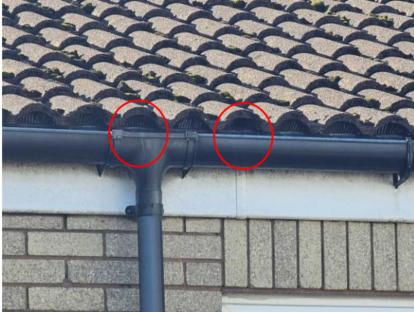
Photo 7: Interlocking tiles with missing wildlife spikes
