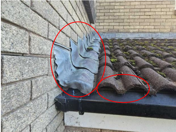
Photo 9: Lifted led flashing and missing wildlife spikes
