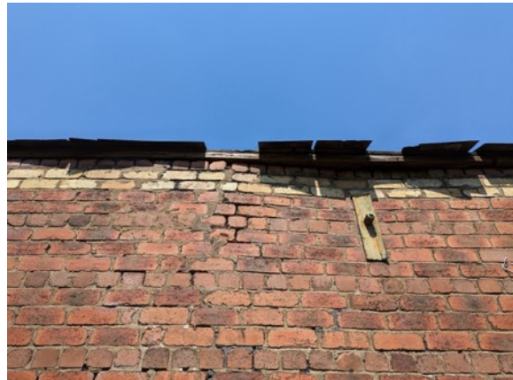
Plate 4: Tiles missing and cracks where mortar missing.
