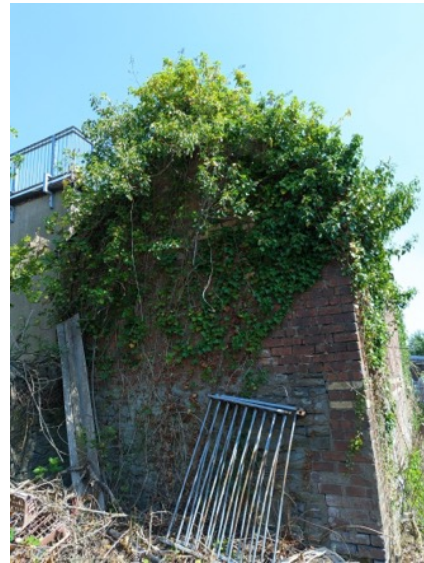
Plate 6: South-west elevation with ivy growing.
