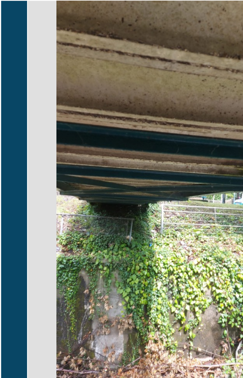
View from underneath the bridge - horizontal cracks in the concrete can be seen.
