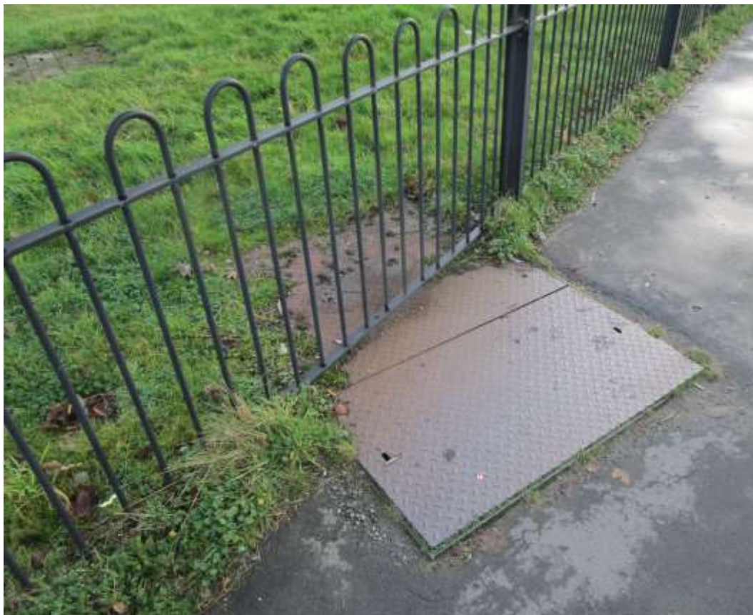
22. Utility cover straddling Hafod land and footway of Pant Rd
