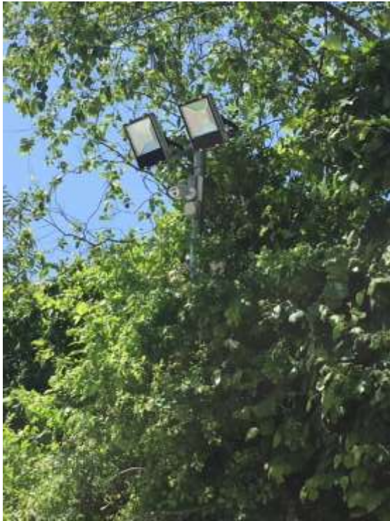
5. Lighting column site H
