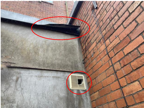
Photo 13: Lifted Metal Trim and Broken Vent Guard on Eastern Rear of Main Section of B1
