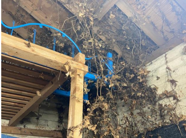
Photo 26: Example of Large Gaps With Vegetation
