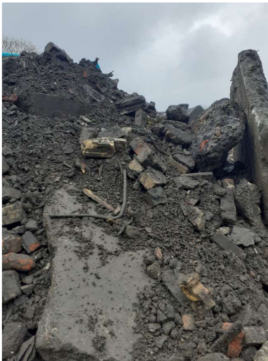
Plate 18: Fragments of rebar, concrete slab, brick, plastic, and tile.
