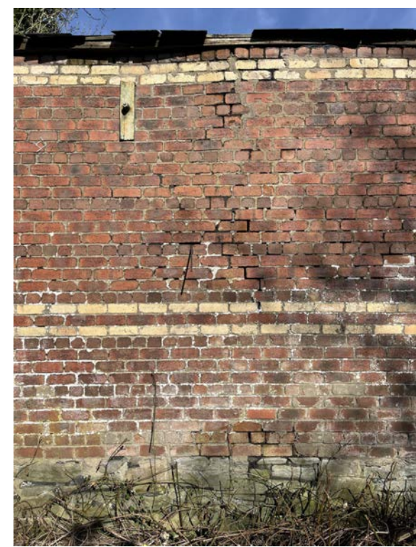
P4 Southeast elevation view showing the movement in the wall, missing gutter and structural tie.
