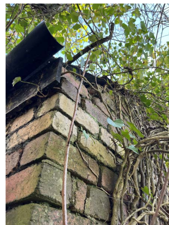
P11 West corner showing the poor condition of the rainwatergoods and roof.
