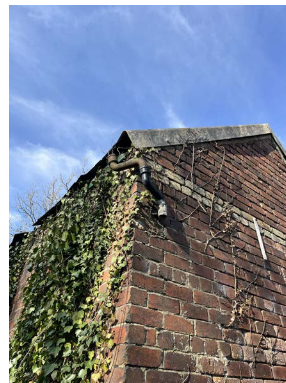
P2 Northeast corner showing the poor condition of the rainwatergoods and roof.
