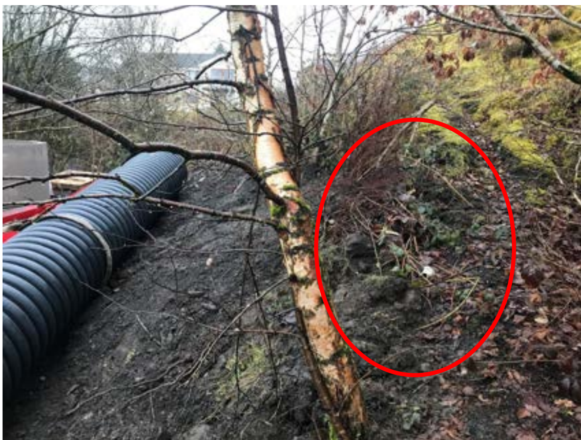
JK3 – scattered viable knotweed rhizomes, etc. across area. Surface shoots placed in circled area, rhizomes seen throughout working area.
