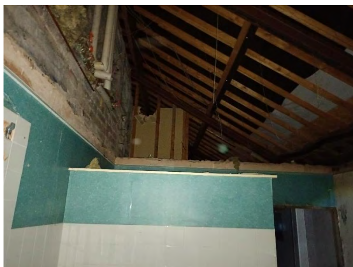
Plate 4-View Looking Up at Ceiling From Room G-Exposed Roofing Felt/ Battens and Joists
