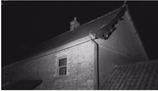
Plate 17: House, infra-red image of north-western gable
