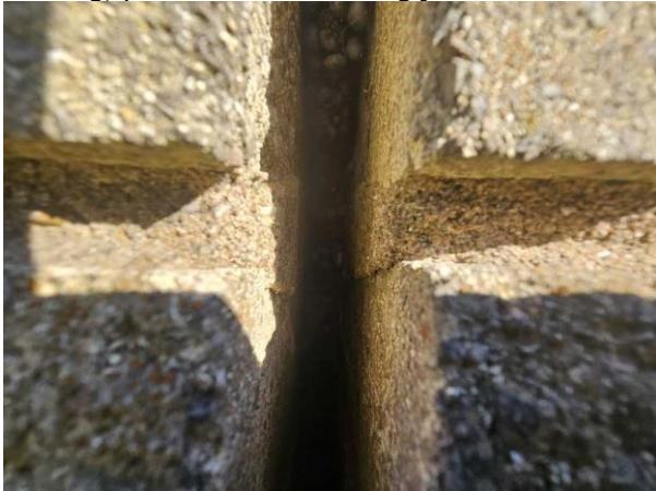
Photo 11: Long gaps running the height of the building, present at the building joins
