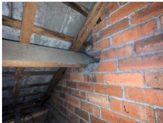
PRFs – Cavity above bitumen membrane.
