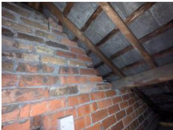
PRFs – Cavity above bitumen membrane.
