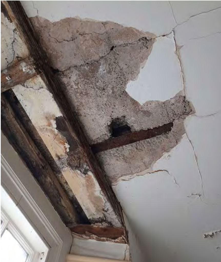
Image from opening up works showing corroded condition of existing steelwork. New steels have been designed to keep depth to a minimum and ensure interventions sit above the window reveals.
